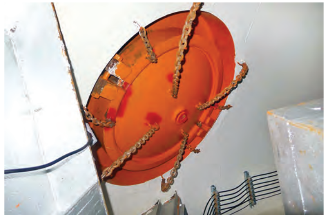
Emergency escape hatch in D-1 LCC. The hatch would be opened with a spanner via the nut in the centre of the hatch
